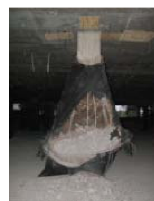
b) Parking garage 1st floor column after explosion
