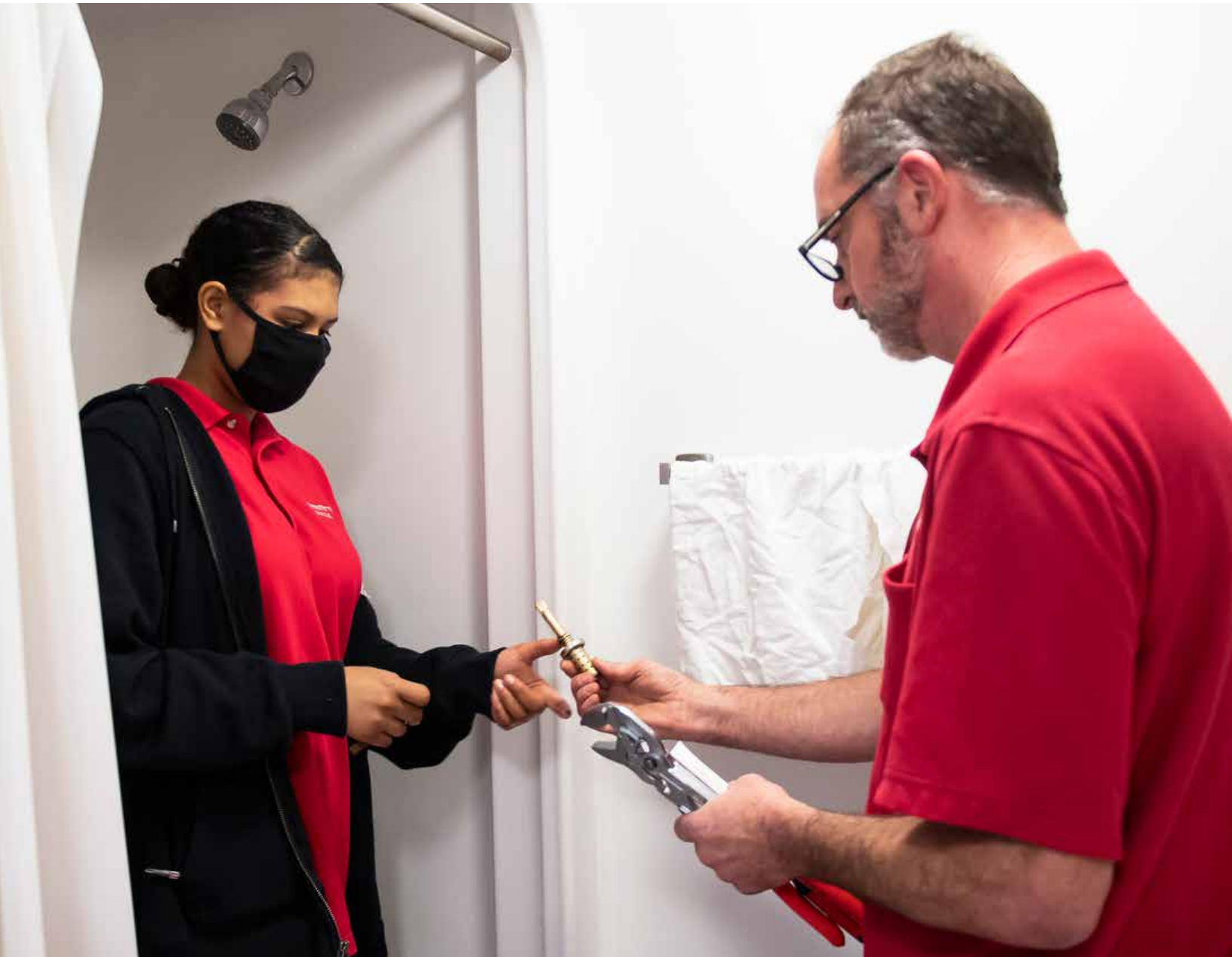
Northeastern University plumber Mike Frost assists Olivia Genera, a Madison Park Technical school student who is working as a plumbing apprentice on campus at Northeastern University, while she works on a shower in the East Village dormitory on Tuesday, June 15, 2021. Photo by Alyssa Stone/Northeastern University. More on Page 11
